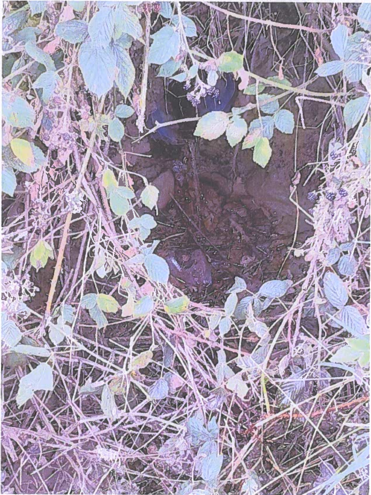
Exhibit P4-3 – Discharge pipe near dwelling house at REDACTED REDACTED on 24 August 2022. Strong Ammonia odour noted at this location.
