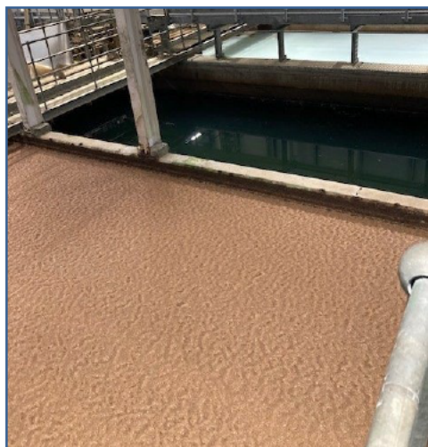
Figure 2 - 1 DAF Cell Sludge Blanket
