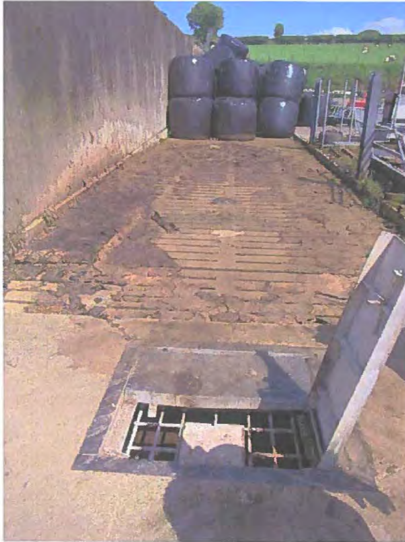
Dried slurry on the slats of the below ground slurry store.
