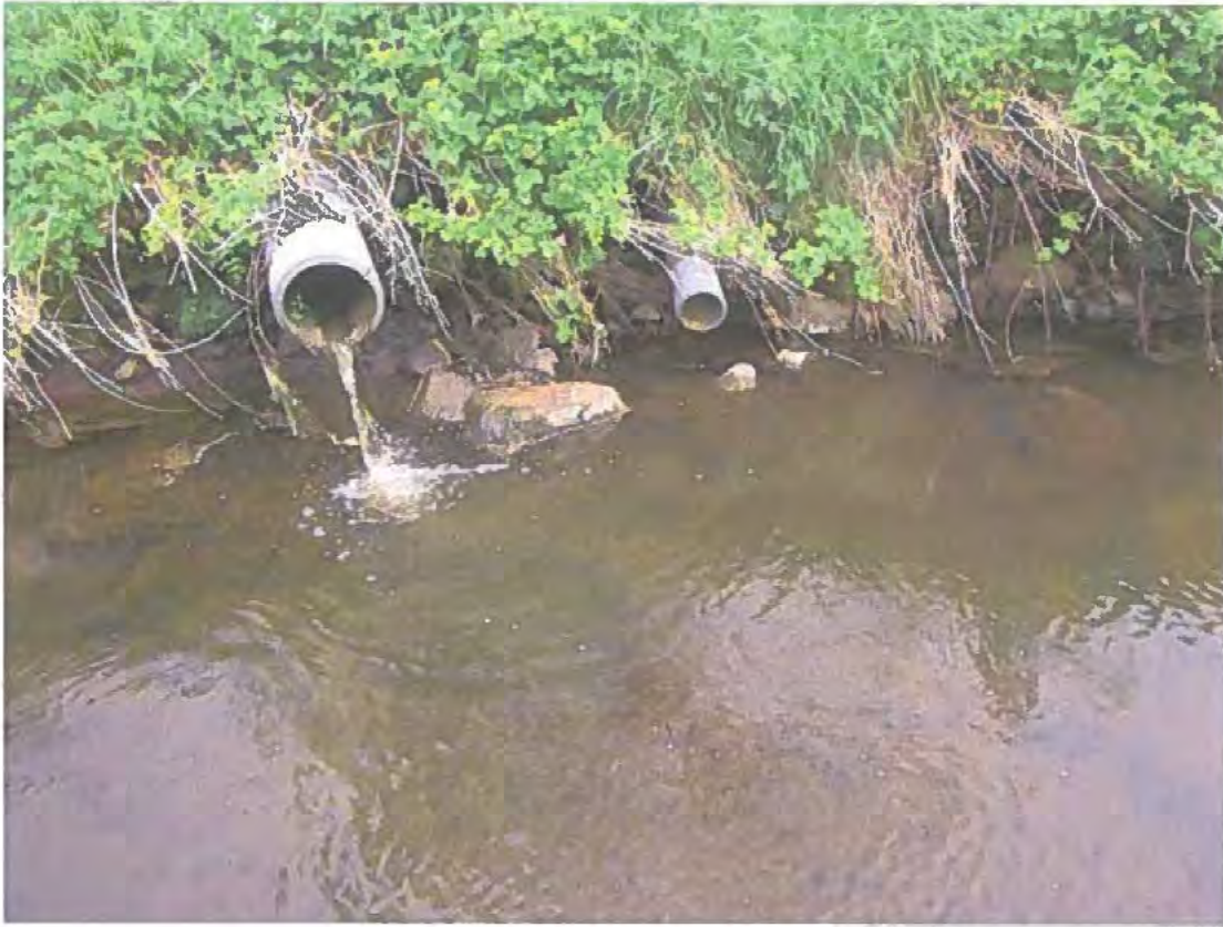
Pipe actively discharging weak dilute slurry to the Ballyclover Burn at [REDACTED] Statutory sample WR3/24/0504 was collected from this location.
