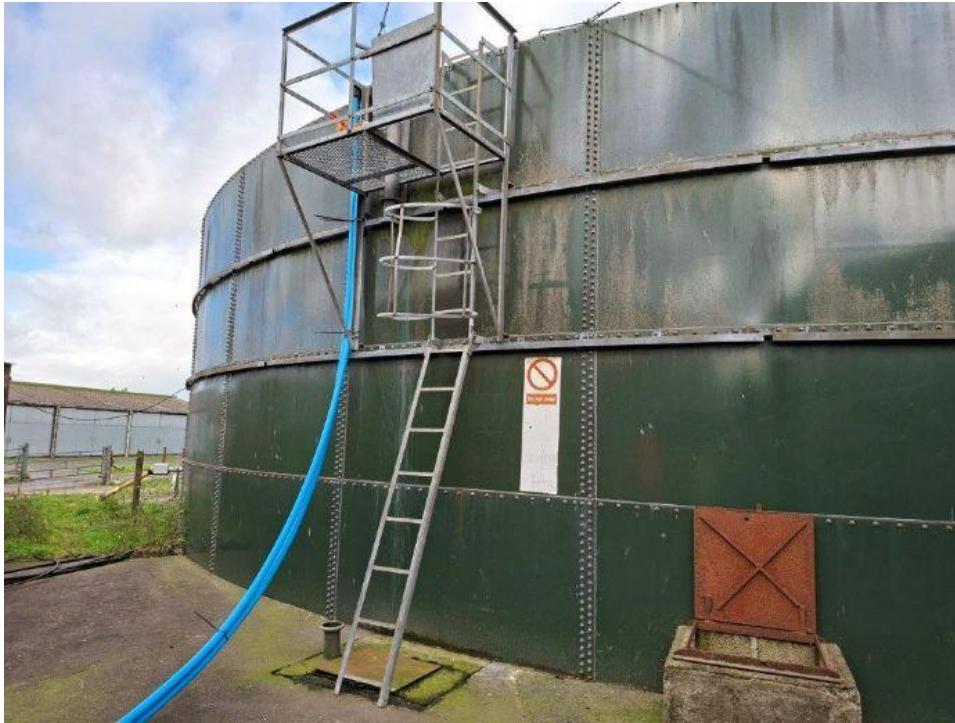
20251028_121811 Dirty Water Tank
