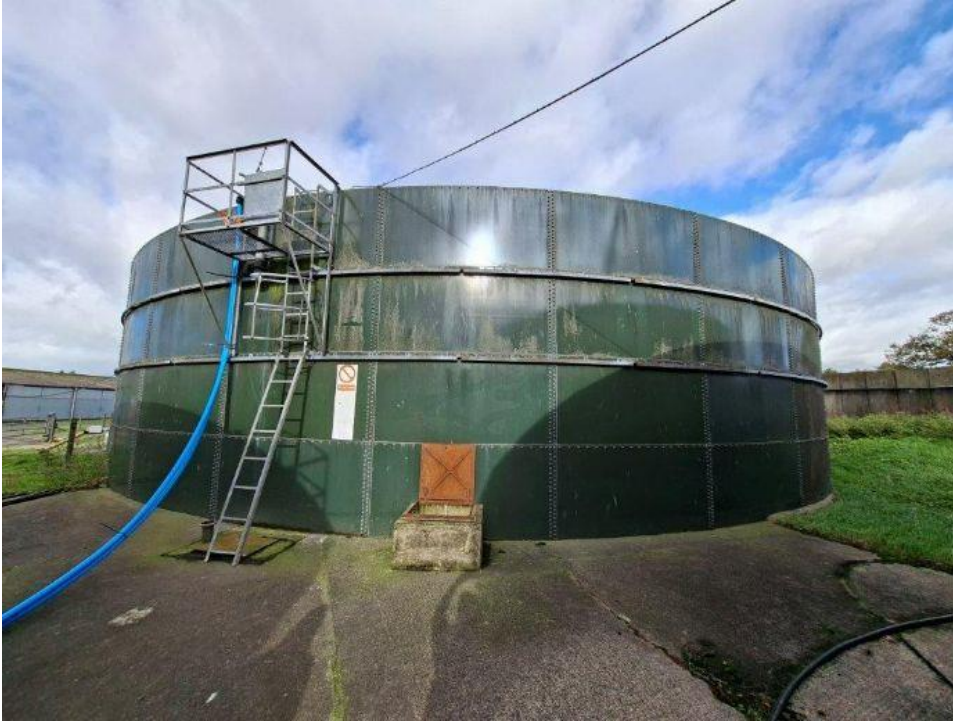
20251028_121714 Dirty Water Tank
