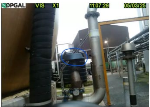
Gas bag PRV Emission location
