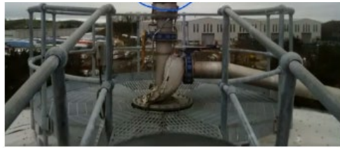
Top of Digester 1 roof PRV Emission
