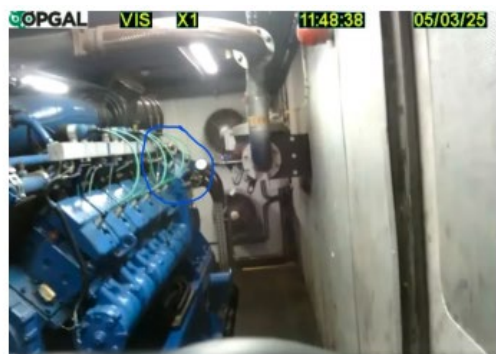
Inside CHP 1 emission location
