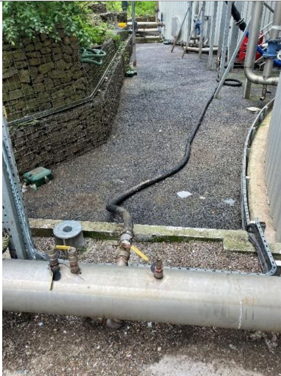
Photo 13 Waste build up around outside tanks
