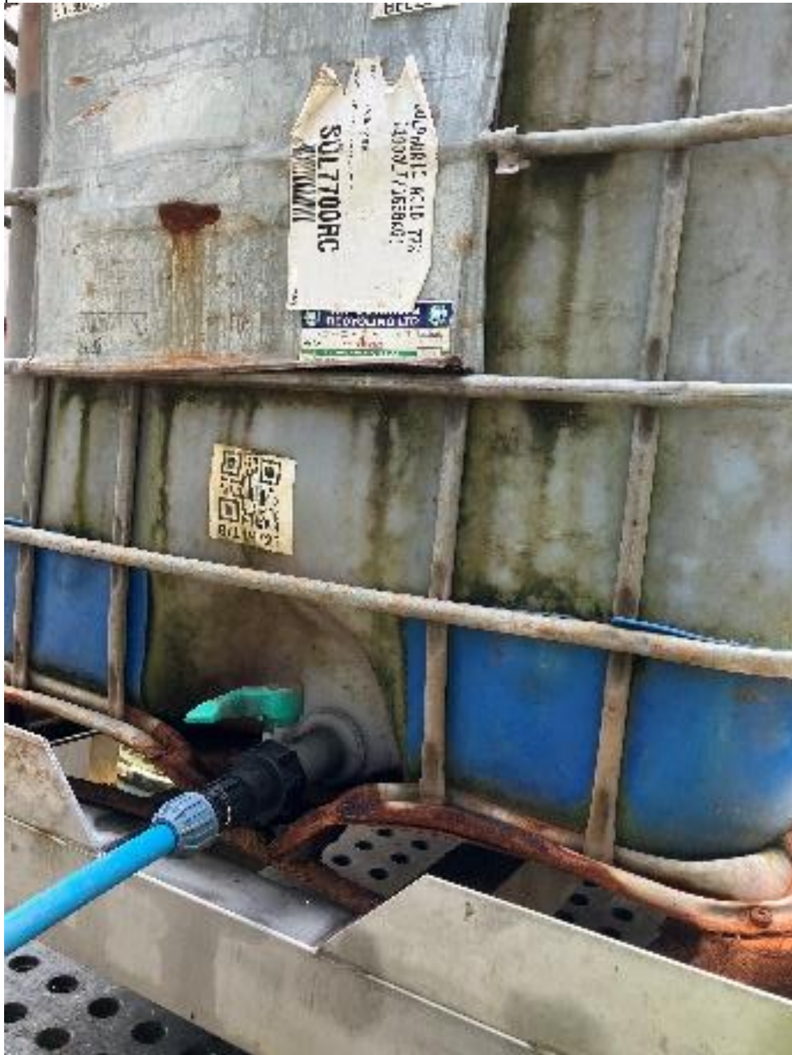
Photo 14 Scrubber chemical IBC
