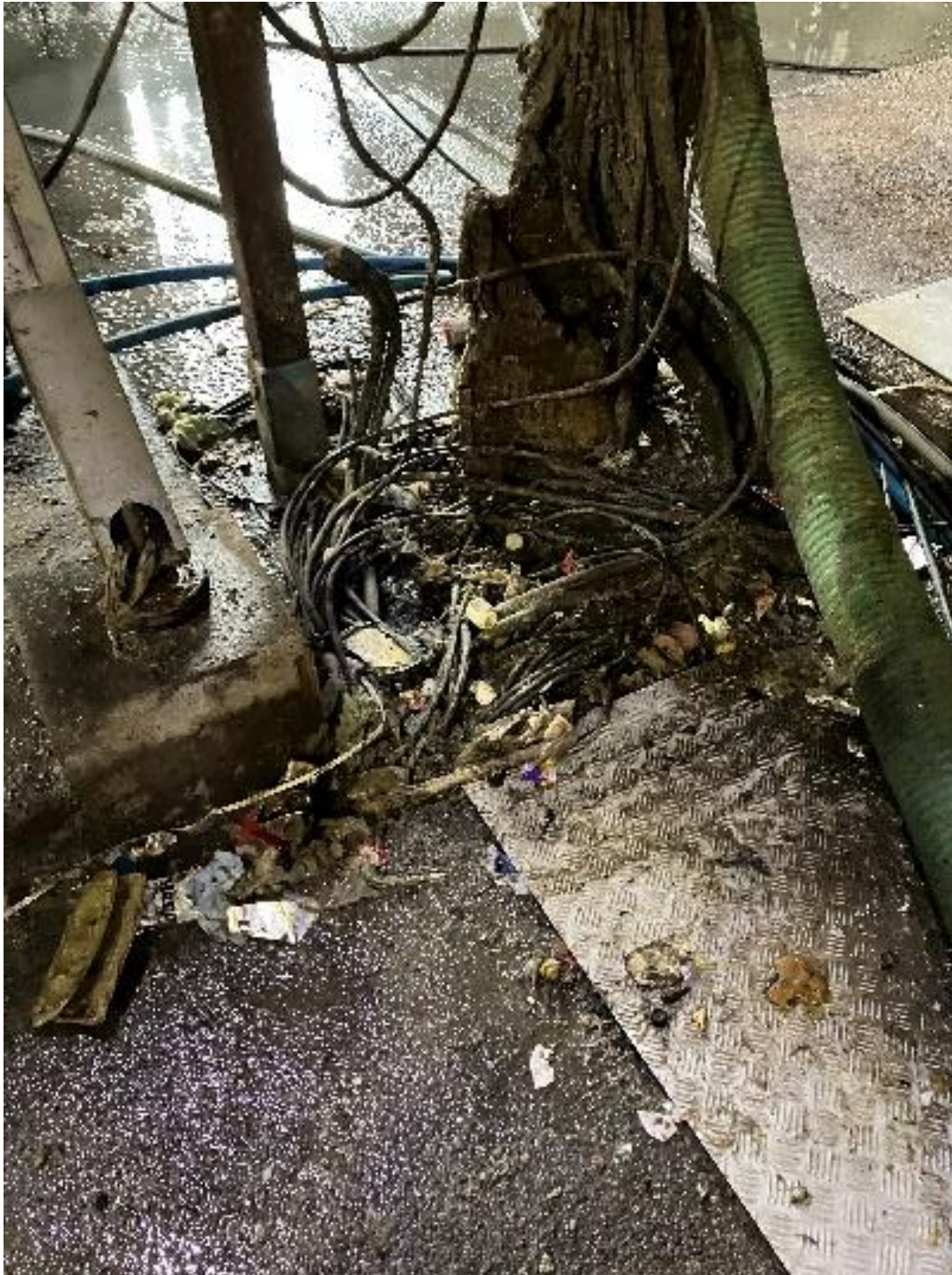
Photo 9 Waste build up
