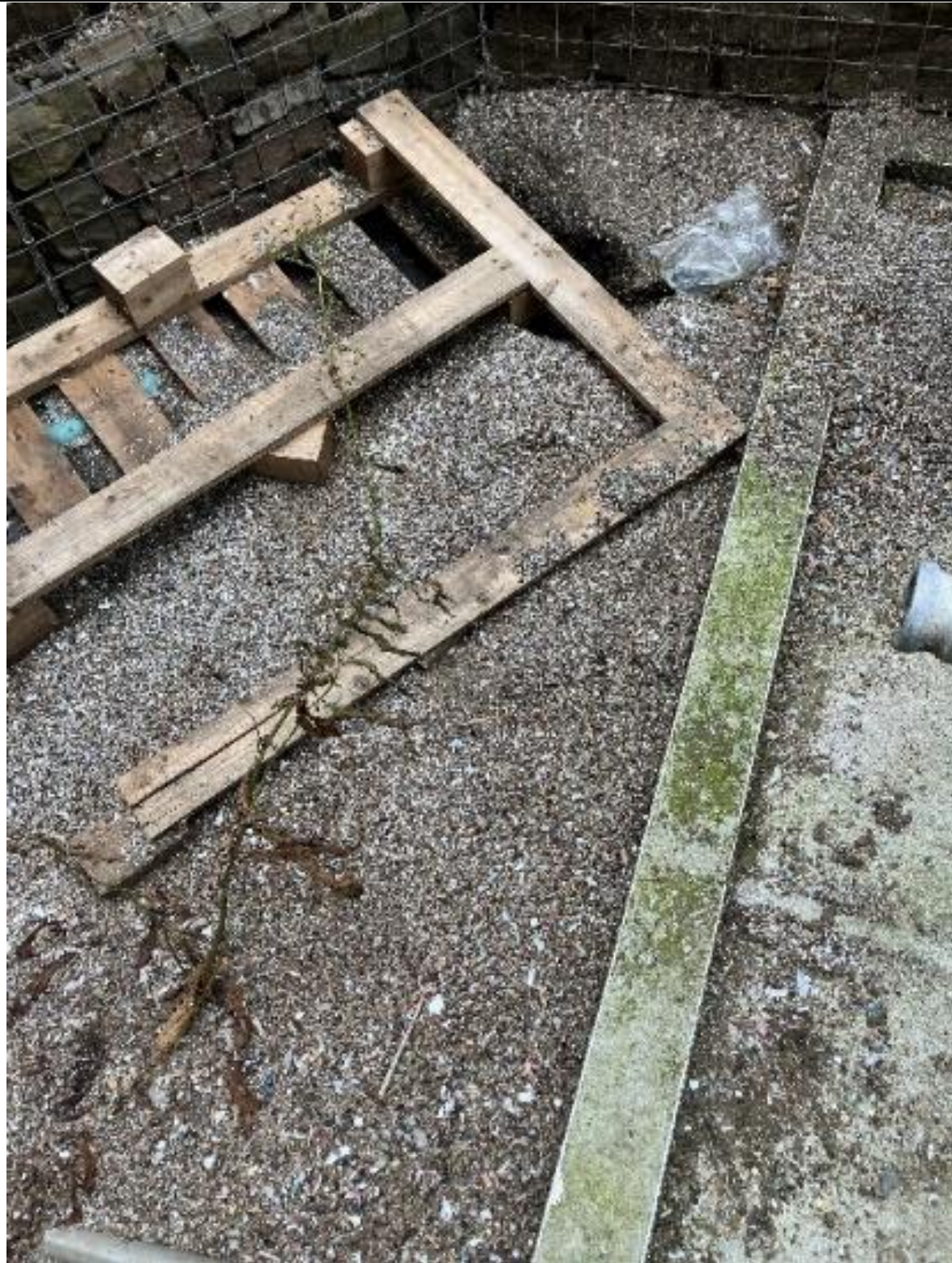
Photo 12 Waste build-up around outside tanks
