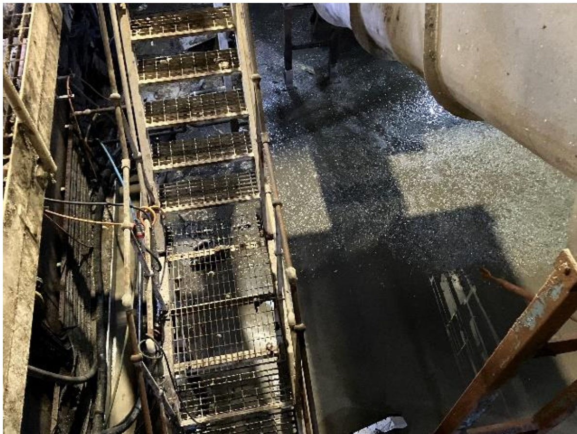
Photo 6 Dirty stairwell and floor area
