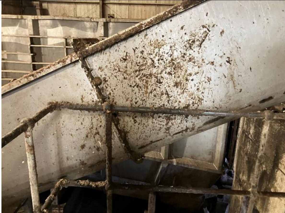
Photo 5 Waste transfer machinery
