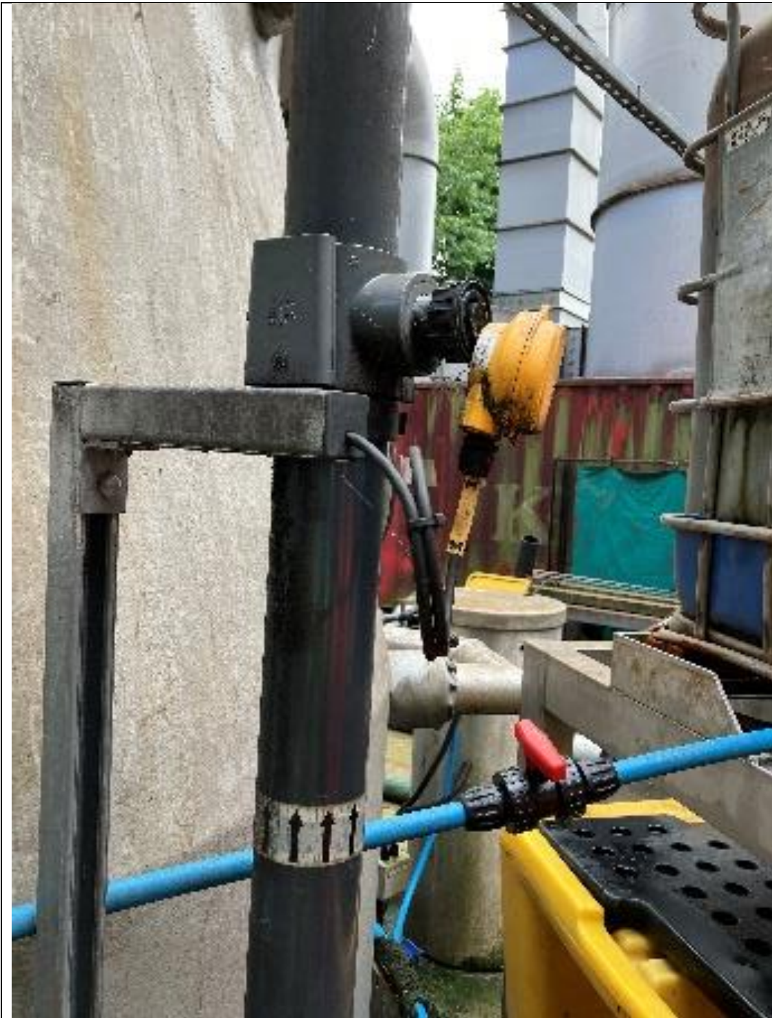
Photo 15 Scrubber chemical dosing
