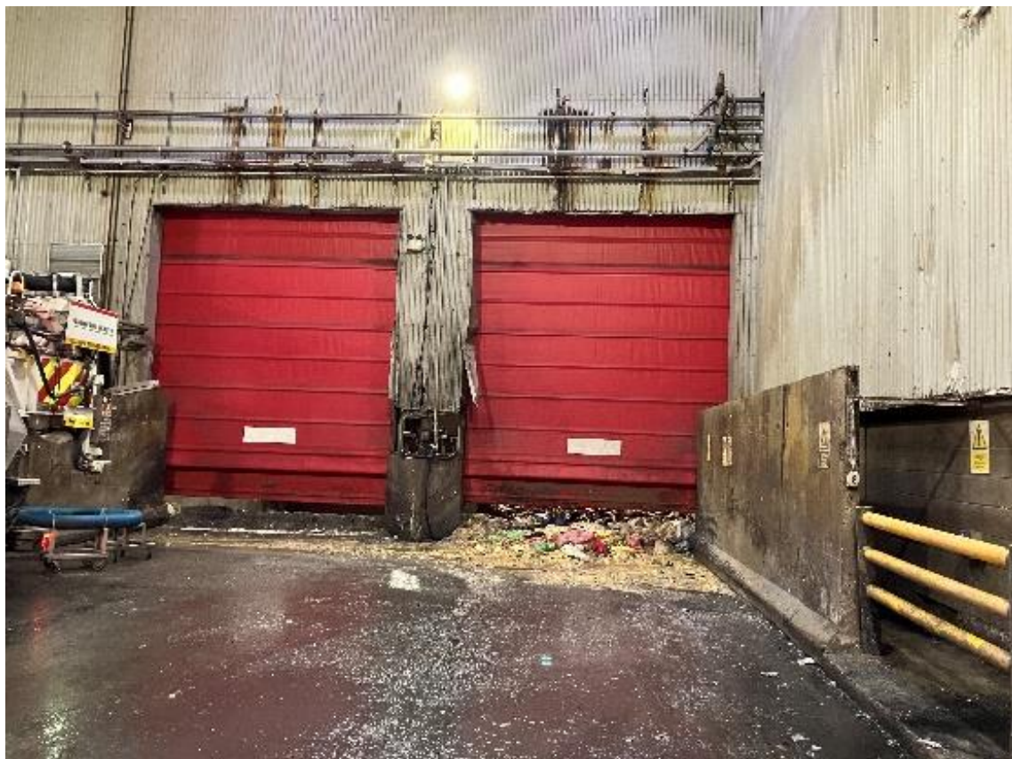
Photo 2 Overflowing waste reception bays
