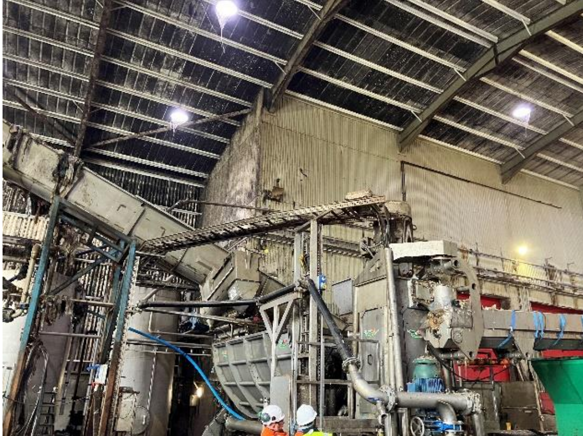
Photo 7 Waste sorting machinery
