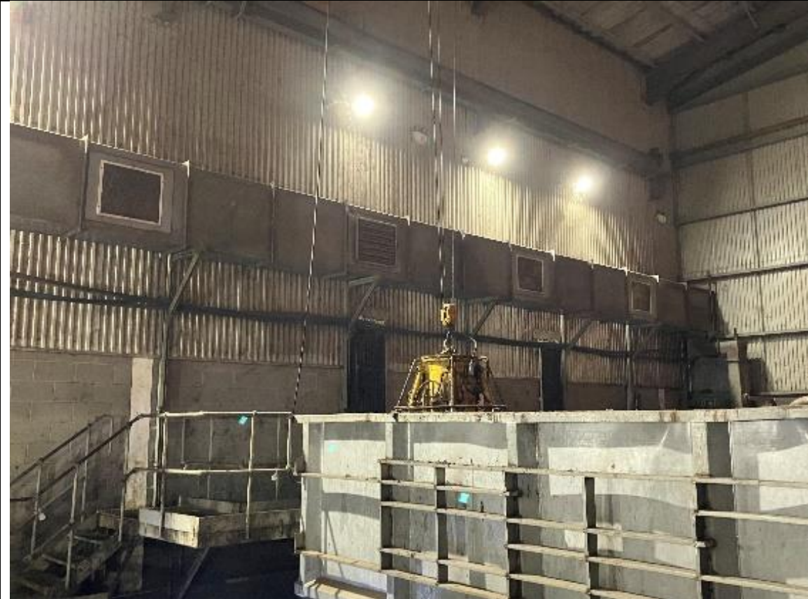
Photo 4 Extraction in waste reception building
