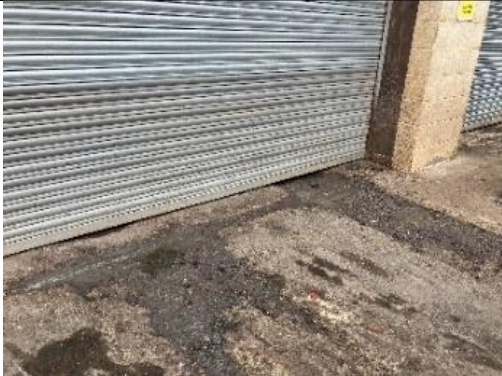
Photo 1 Rubber seal missing from bottom of doors in waste reception building
