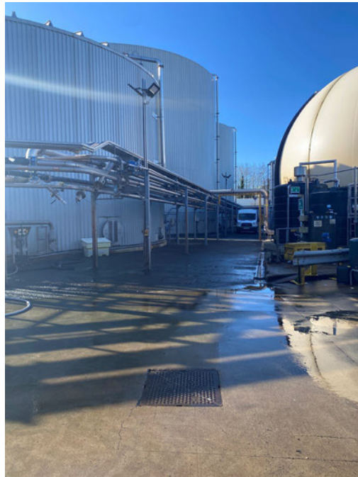
Photo 7 Digestate tanks and gas balloon
