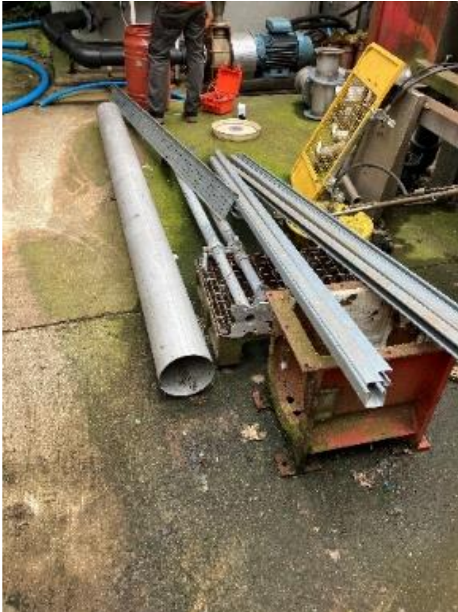
Photo 16 Waste build up in scrubber area
