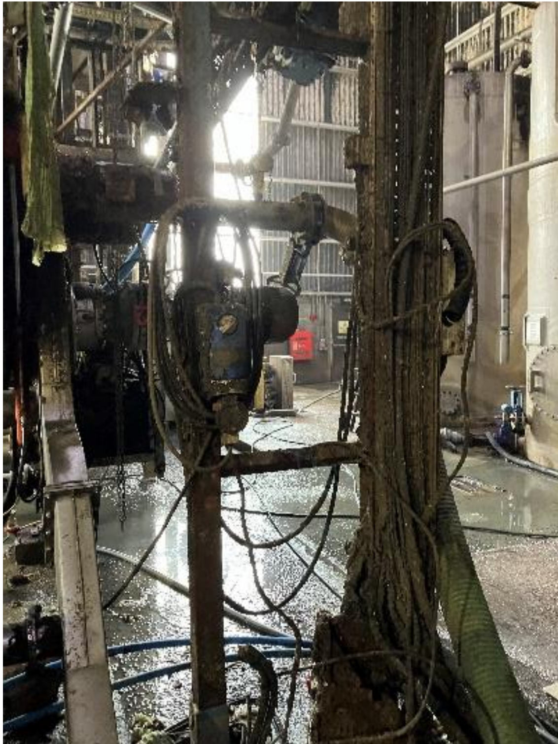
Photo 10 Dirty, waste covered floors
