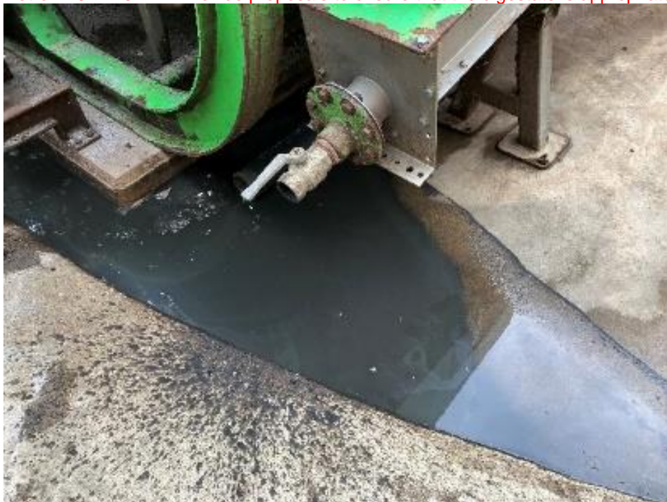
Photo 19 Build up of contaminated liquid beside digestate screener
