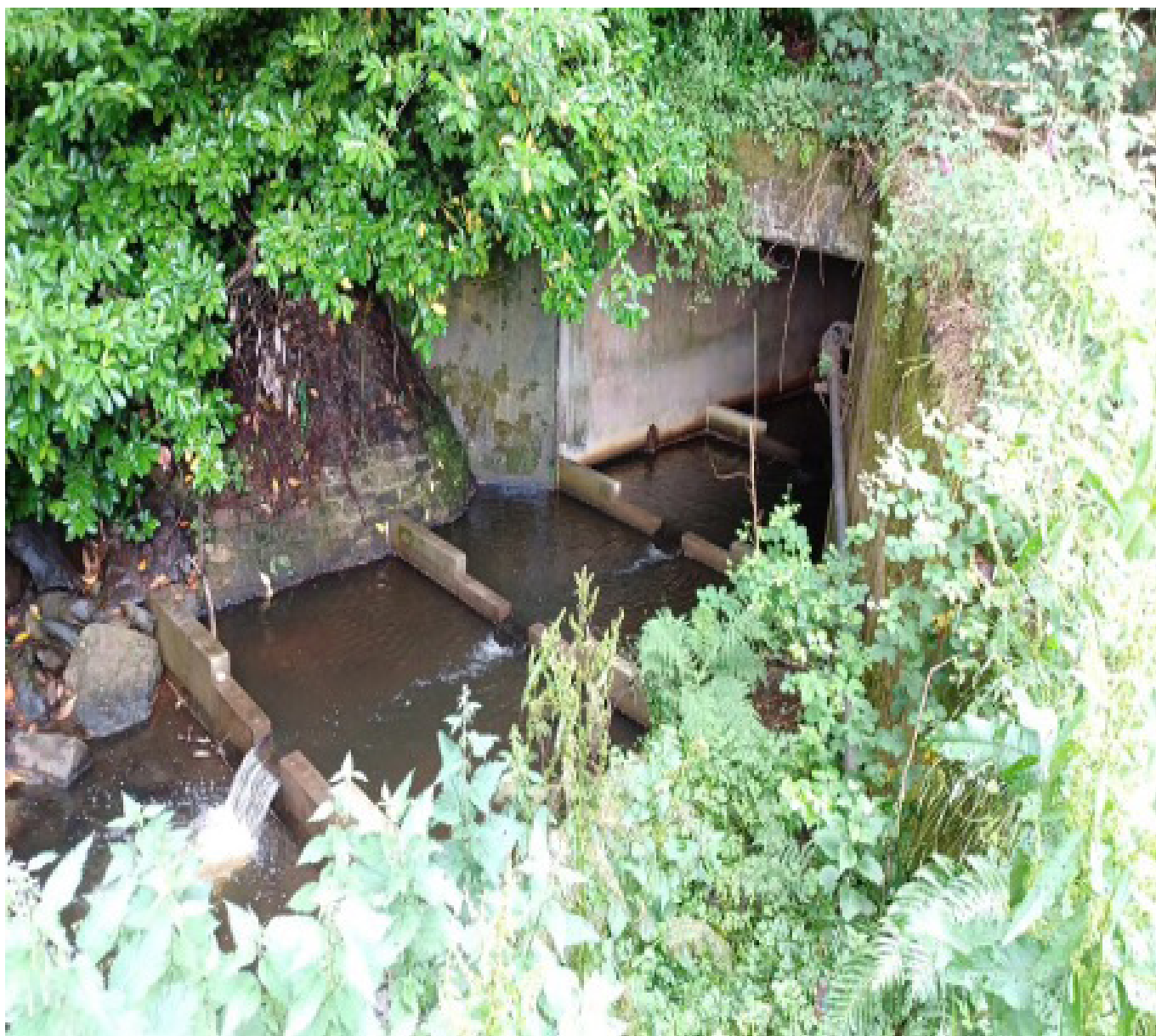
Image showing stepped pools leading to box culvert accommodating fish passage.
