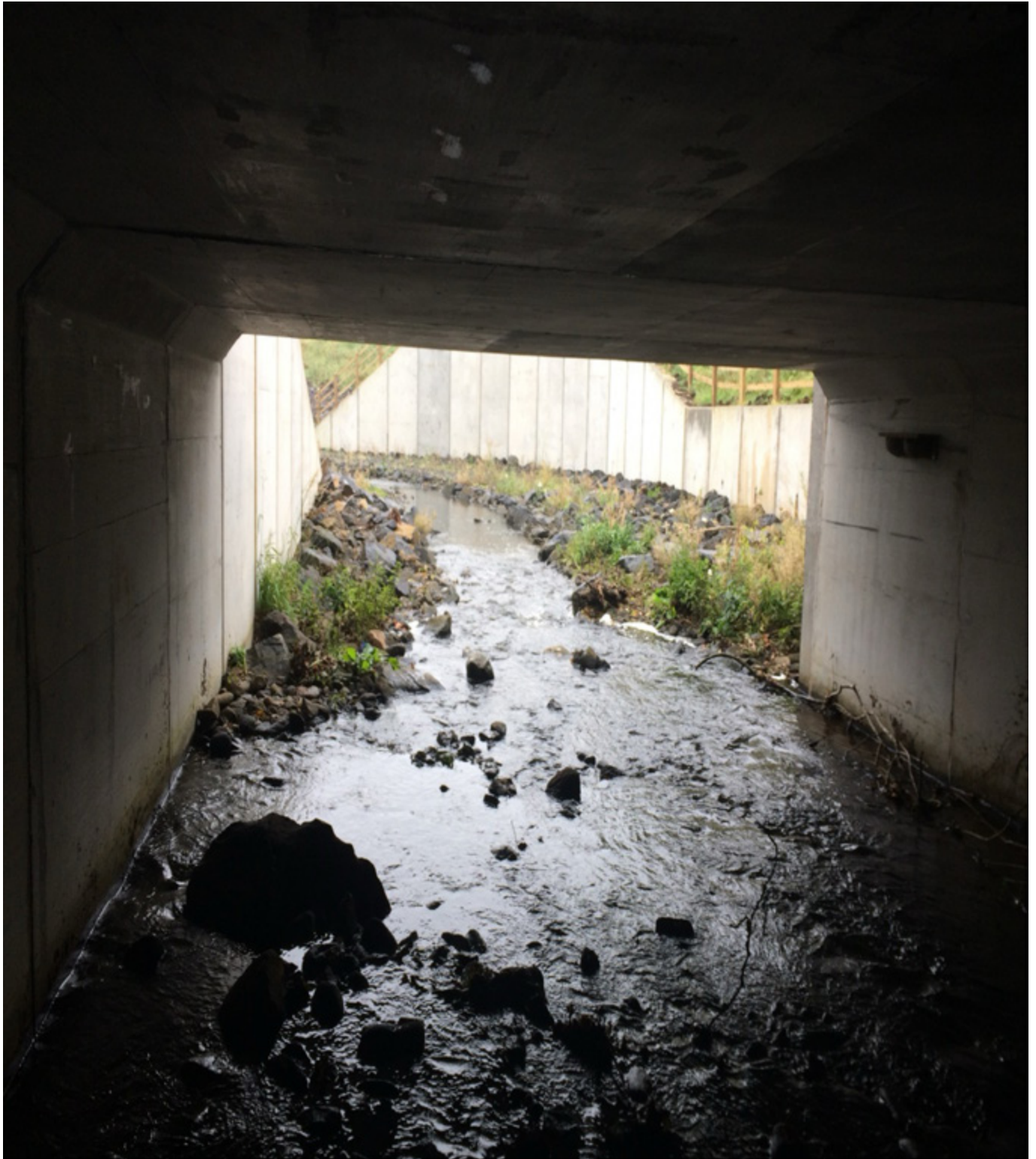
Image showing A31 Magherafelt Bypass culvert with natural collection of bed material taking place towards the culvert exit.
