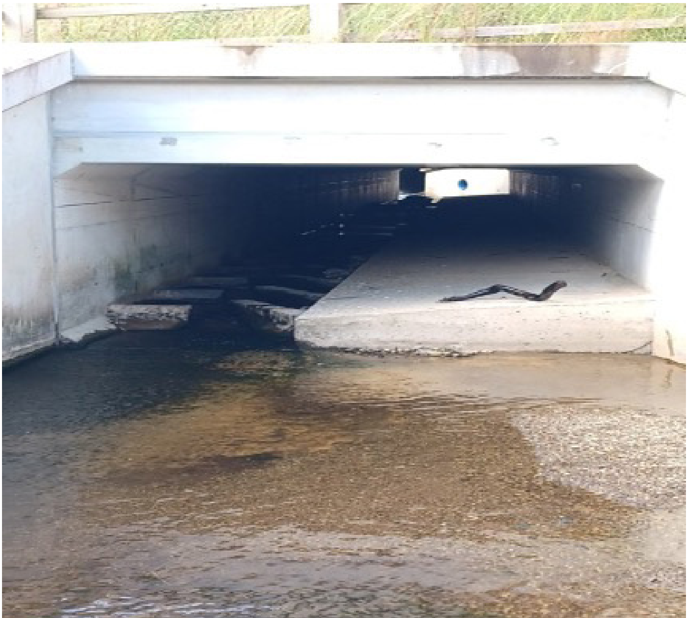
Box culvert accommodating fish passage via baffles and corridor for mammal passage.
