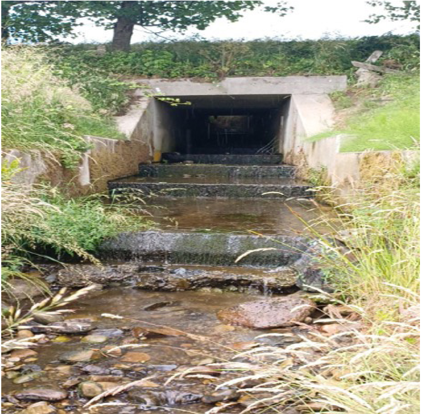
Example of poor fish passage, flow spread across weir crests and no pool for fish to jump from to ascend steps.
