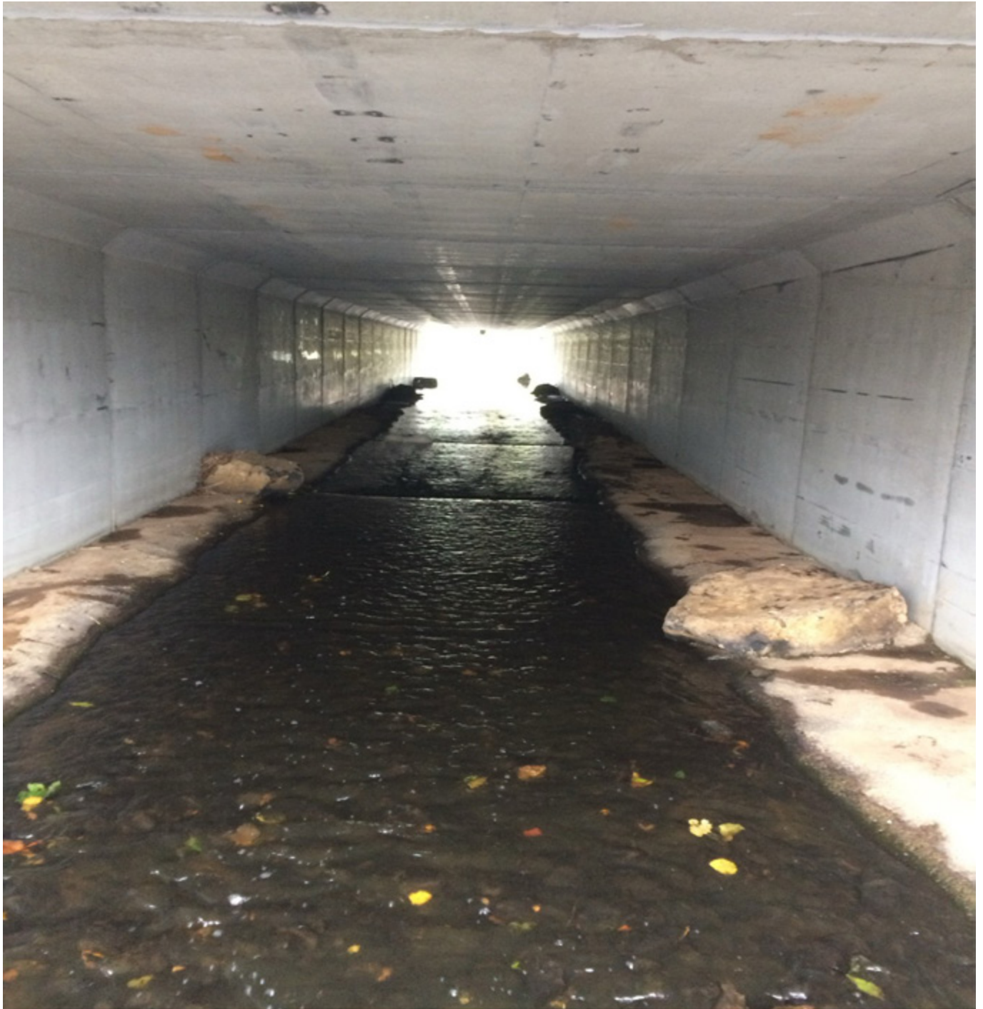
Image showing box culvert on the A4 with precast low flow channel included within the box design recreating the natural channel bed.
