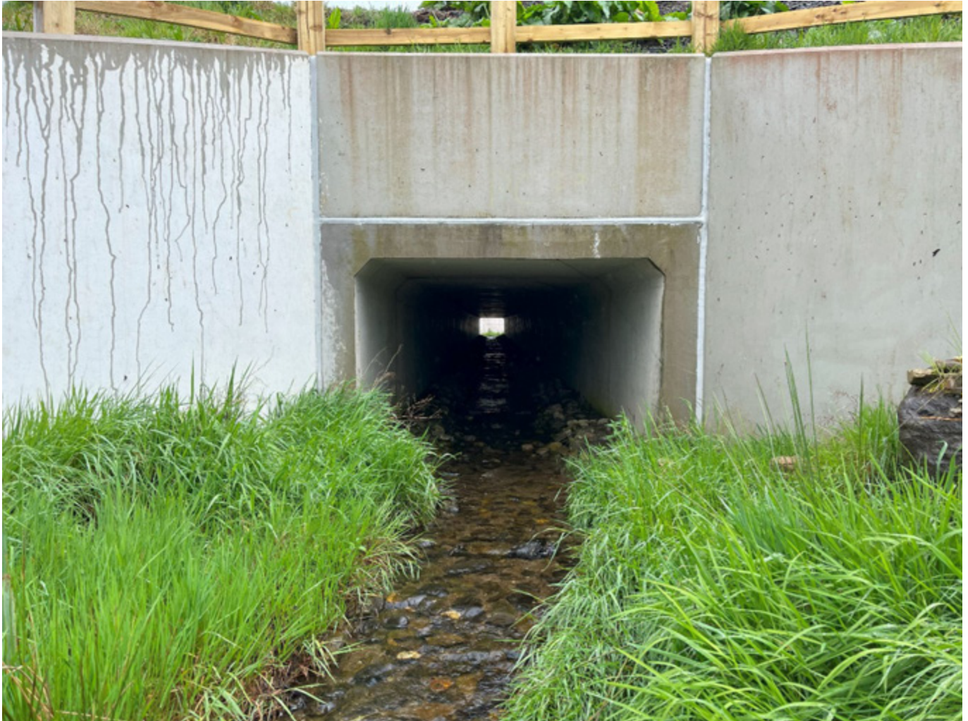
Image showing box culvert from A6. Recreation of riverbed within the vertically over heightened culvert allowing light to permeate throughout.
