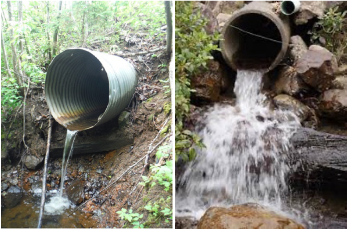
Example of poor design of a 'Hanging Culvert', this has a drop from the outflow to the water below creating a barrier to fish migration.
