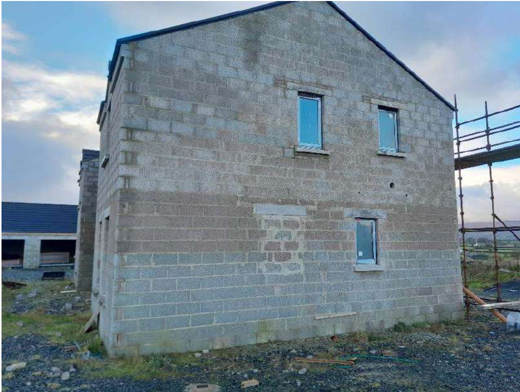
Vent point located at ground level on the eastern side of the dwelling
