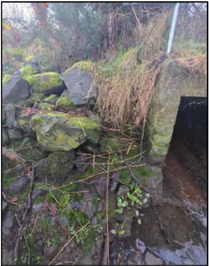
PHOTO 1 - ELEVATION VIEW OF VOID ADJACENT TO CONCRETE CULVERT STRUCTURE PHOTO SOURCE - AMEY (2026)
