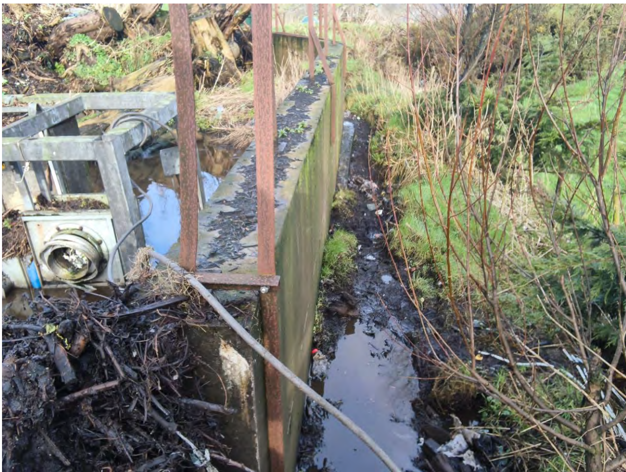
Figure 4 Signs of previous untreated dirty water escaping from site confines.
