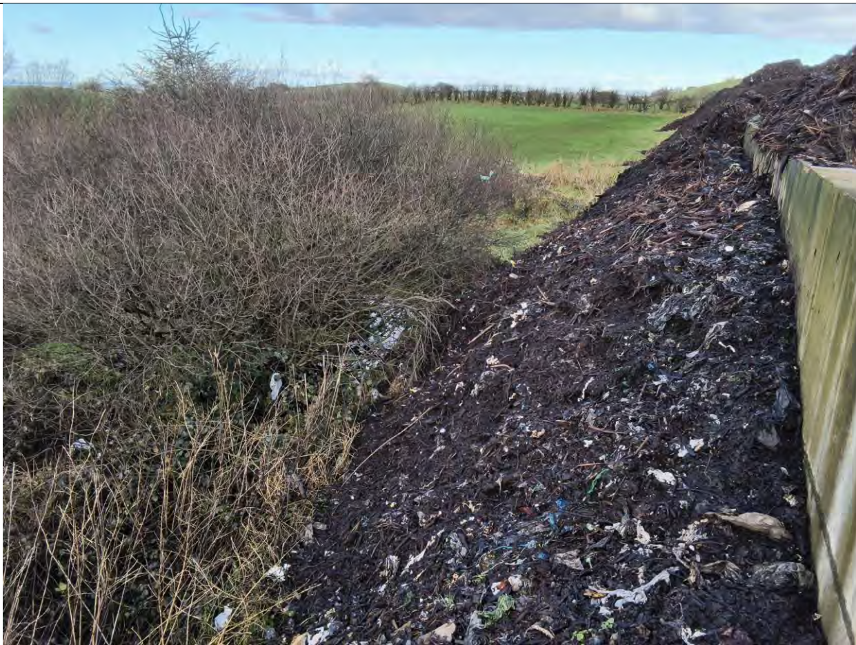
Figure 11 Site material being deposited outside the sites boundary.
