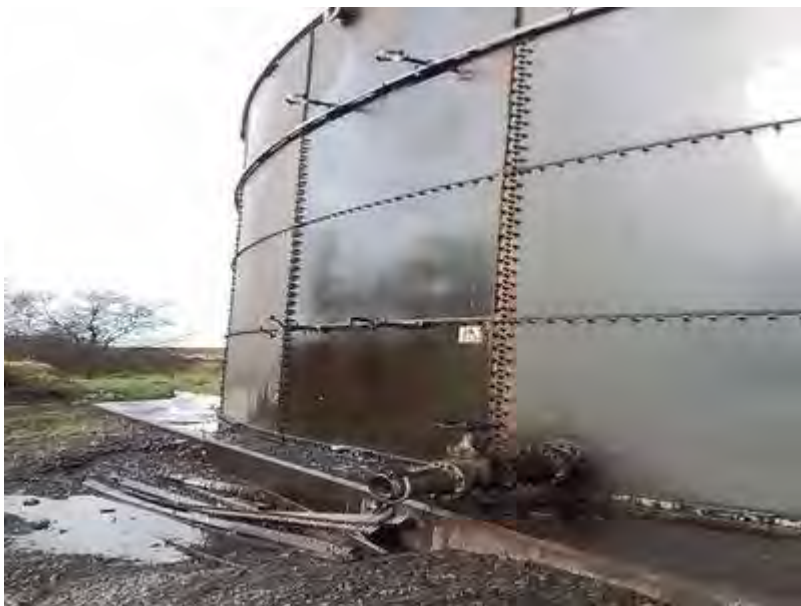
Figure 12 Above ground storage tank with water flowing over the top.
