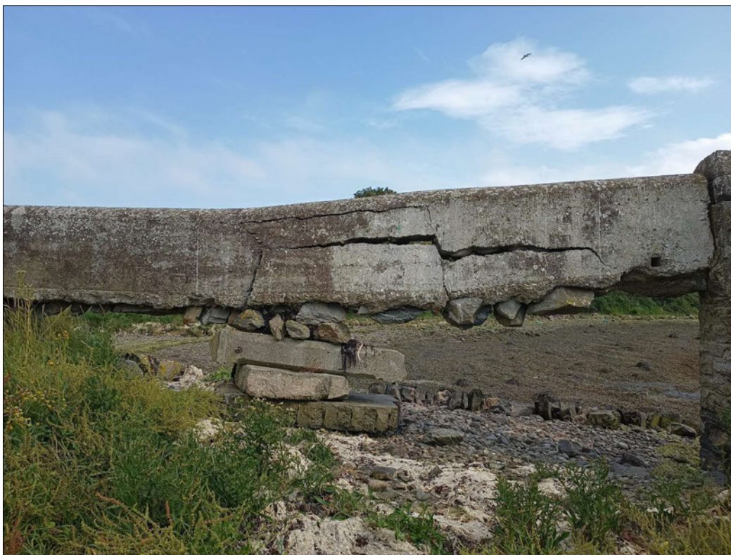
Figure 9: Photograph of the failed parapet suspended between the stone abutments, facing southeast
