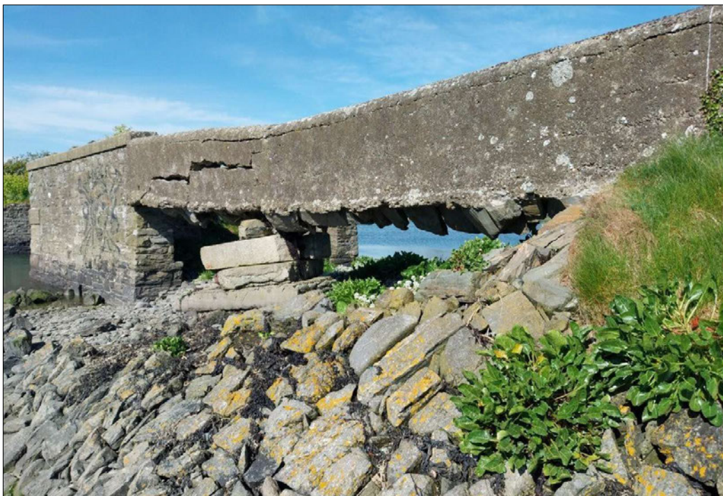
Figure 8: Photograph of the eroded section of embankment/causeway, with the parapets suspended between the stone abutments, facing west (Source: Client)
