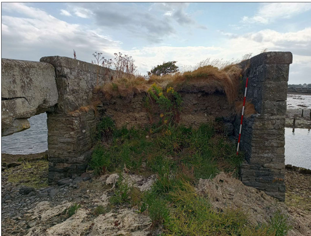
Figure 12: Photograph of erosion within the stone abutment adjacent to the parapet, facing southwest
