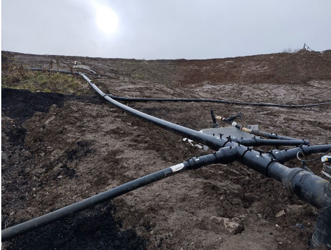
Figure 1.3 – New Gas Line
