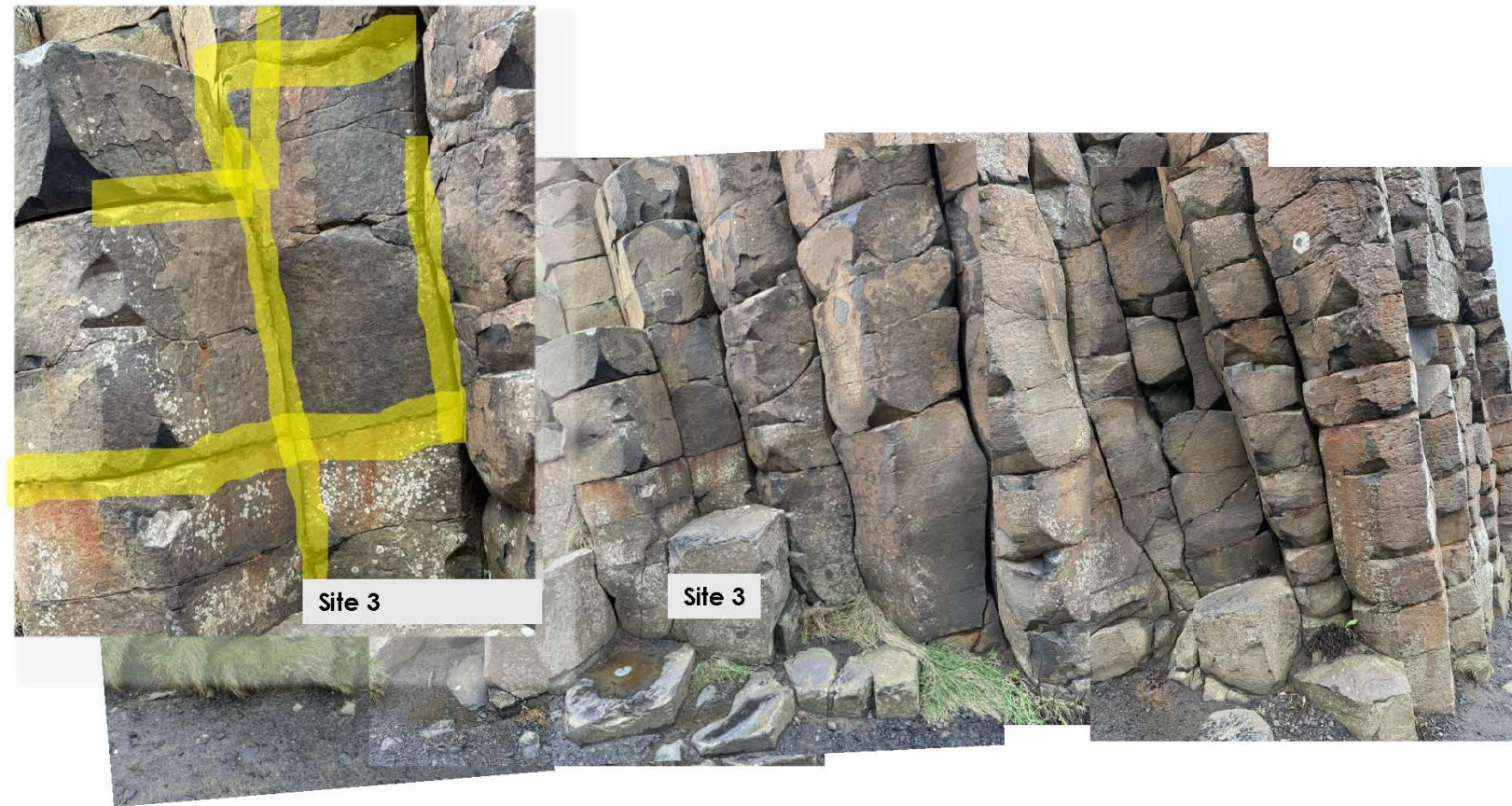
Figure 10. South Elevation (at Gateway) - Inset image shows highlighted joints with coins inserted ~1 linear metre
