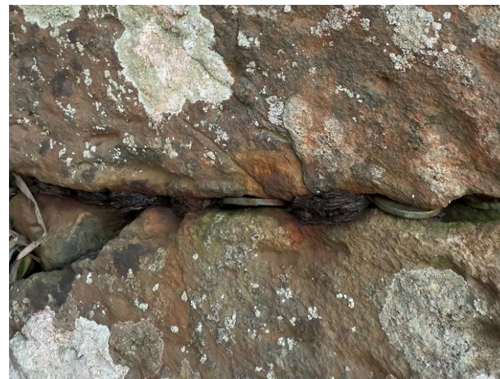
Figure 13. Rusting coins in joints – note expansion of metal on corrosion of some coins
