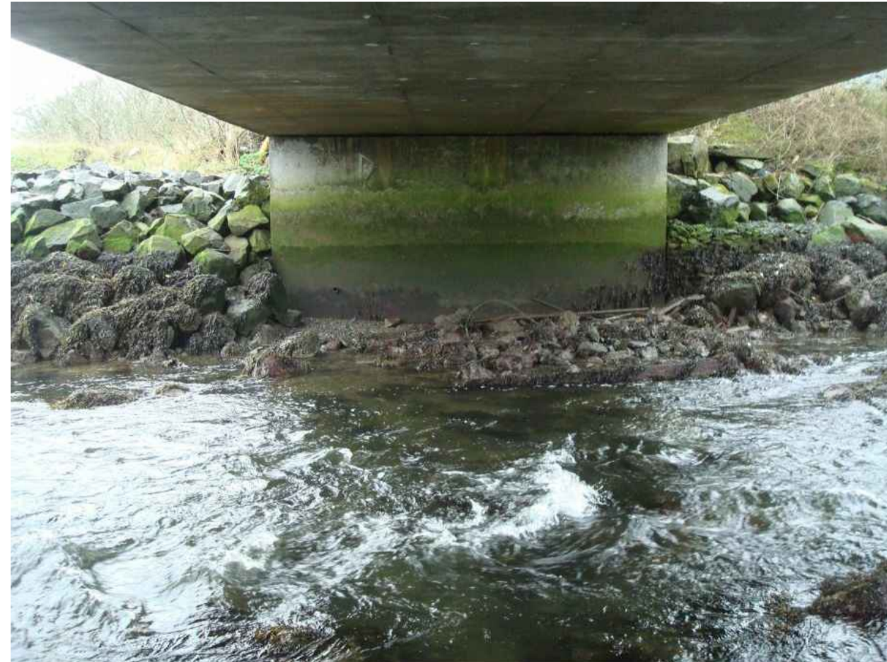
Photo 2 - Loss of rock armour at Low Mileage abutment
