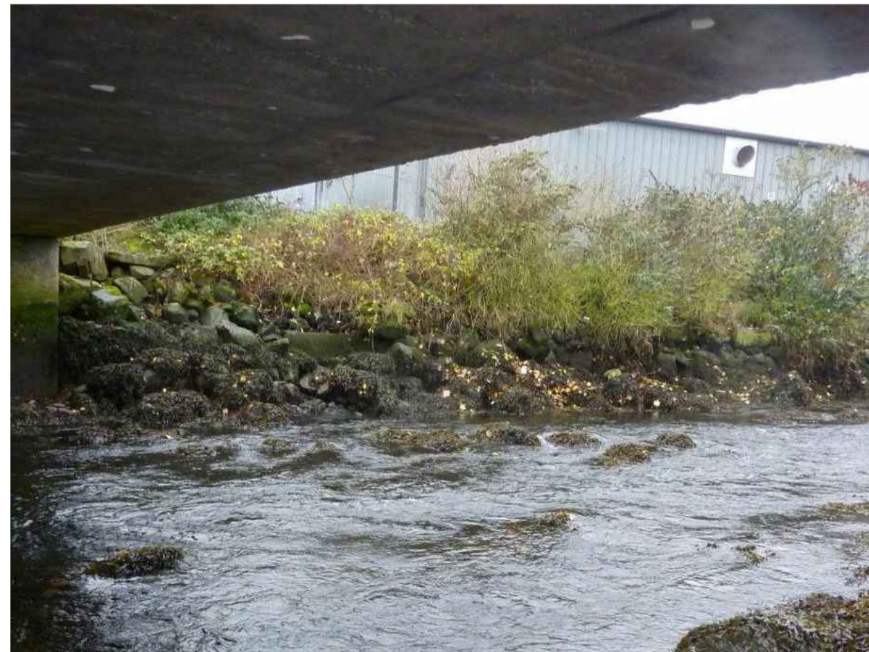
Photo 4 - Loss of rock armour at downside Low Mileage bank
