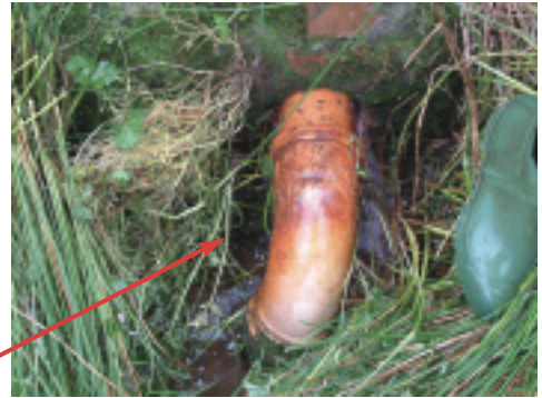
Overflow pipe at source A3
