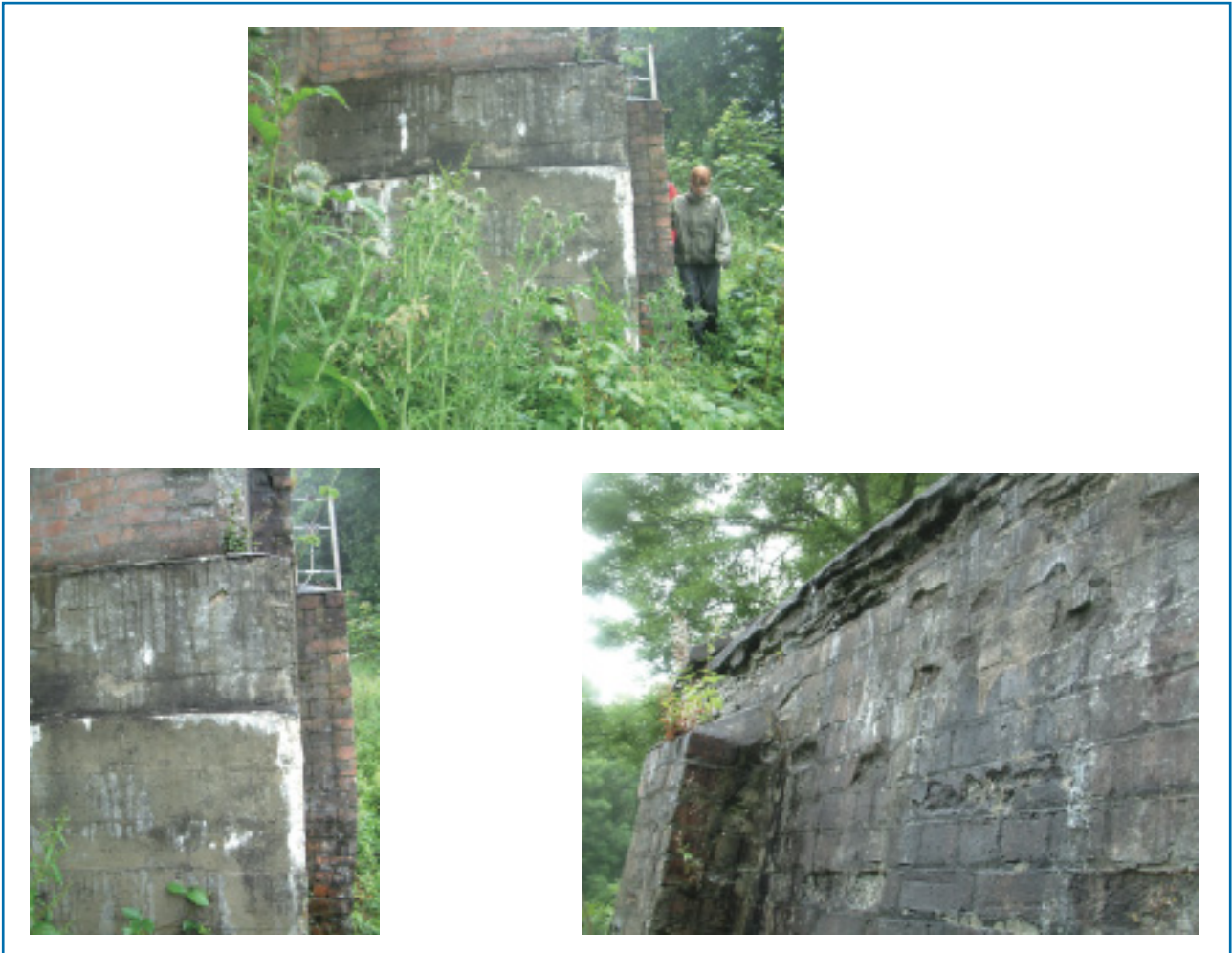
Figure 5.16 Tank B2 showing poor external condition and structural repairs
