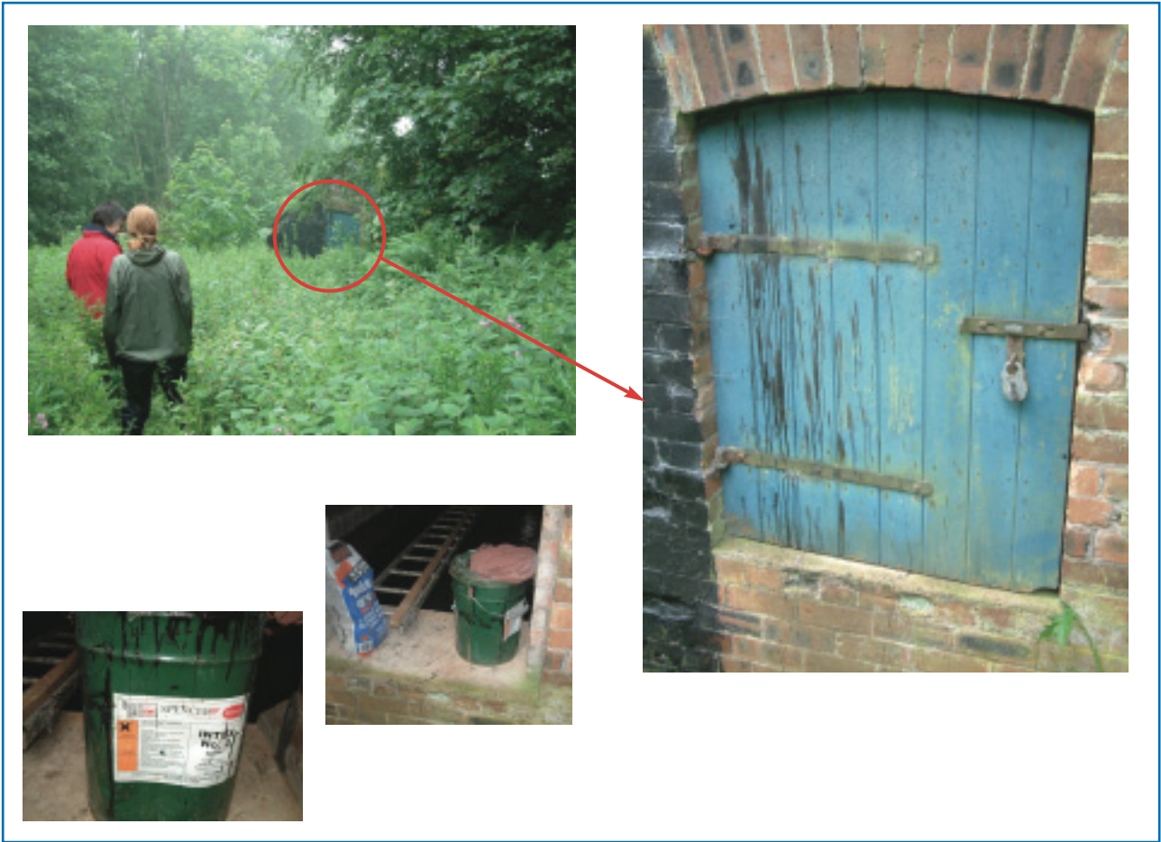
Figure 5.14 Tank B2 showing inappropriate bitumen paint used in internal tank repairs
