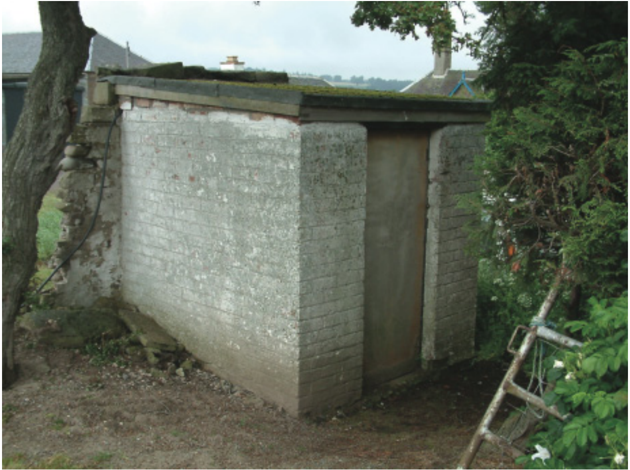
B1 pump house and pressure vessel for Rooster supply
