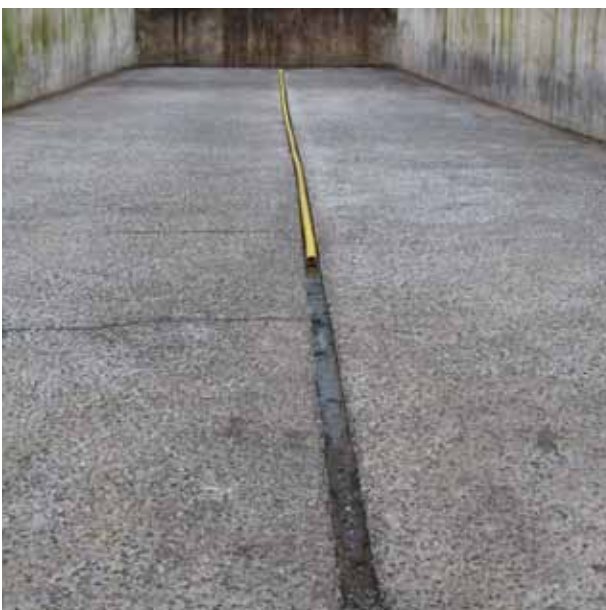
Photo 7: Run-off from an empty and cleaned silo would be clean water.
