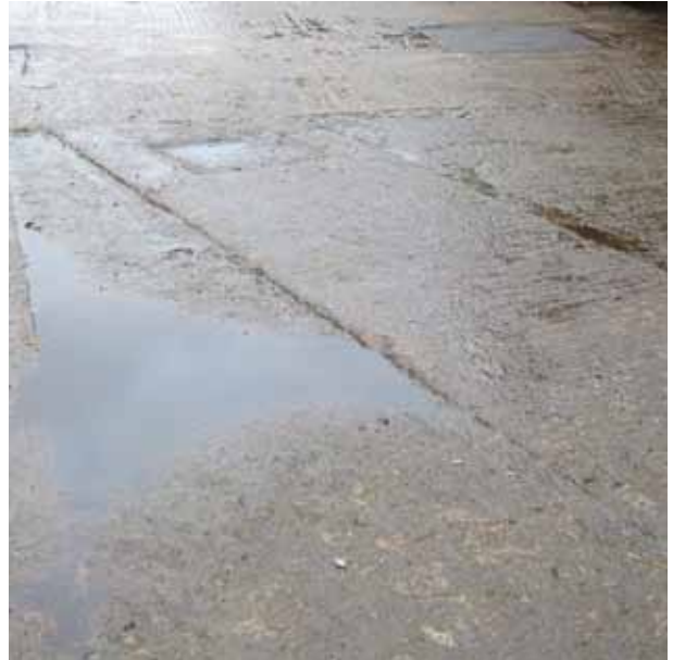
Photo 6: Run-off from a frequently used roaming yard is slurry.
