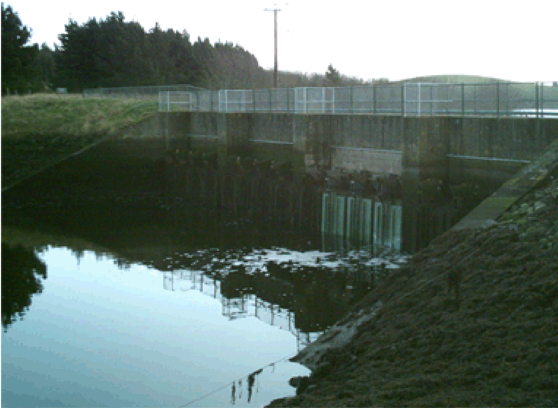
Plate 1 The Quoile barrage at the mouth of the estuary on the River Quoile.
