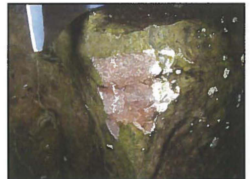
The rock is discoloured from groundwater movement.
