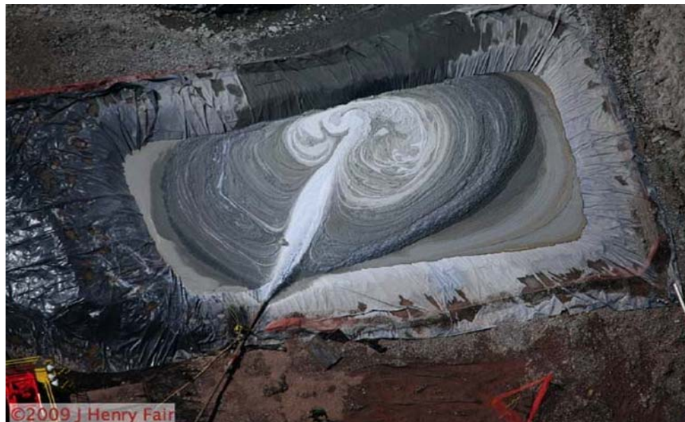
Wastewater flowing into a containment pit (US).
