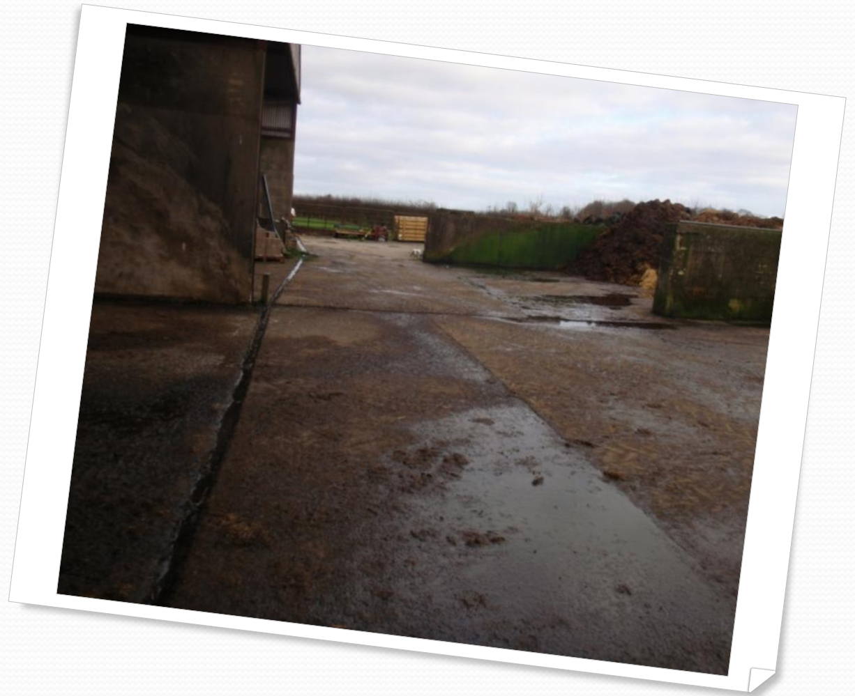
Another overflowing dirty water tank in the Enniskillen sub-catchment
