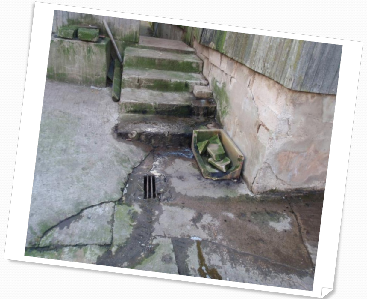
A single block above-ground pig slurry tank. Cracked walls allow slurry to reach the stream.
