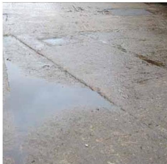
Photo 26 – Run-off from a frequently used roaming yard is slurry.
