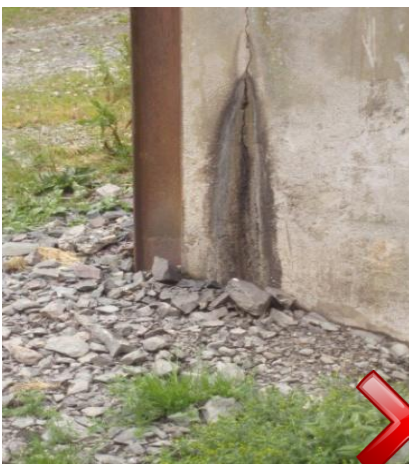
Photo 6 - Leaking silage clamp
