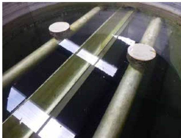
Figure 3.5: New Granular Activated Carbon Filter at Clay Lake
